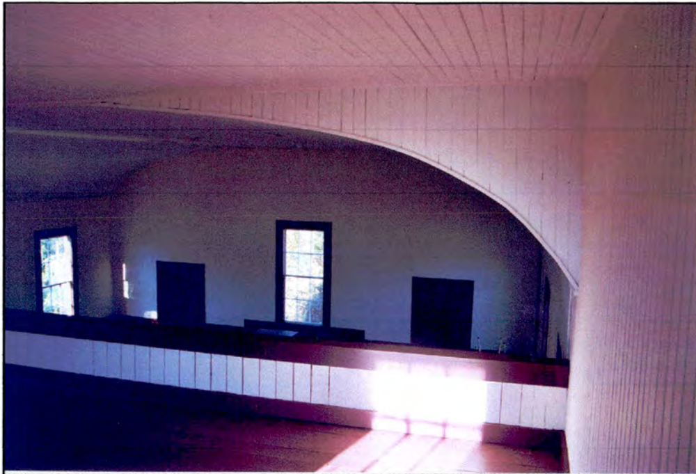
Property 5: Upper Gallery, east wall (n. b. arched ceiling and tongue-and-groove balustrade) ( Figure 20 )
