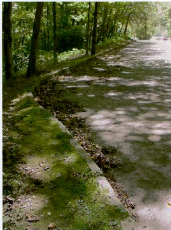
Figure 24. Automobile pull-out, east side Newfound Gap Road near north intersection with Oconaluftee Visitor Center
