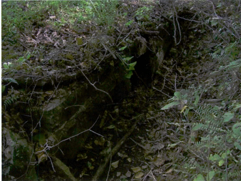
Figure 19. Pipe culvert (Sta 18+00) – east headwall, north of existing and proposed intersection with Tow String Road
