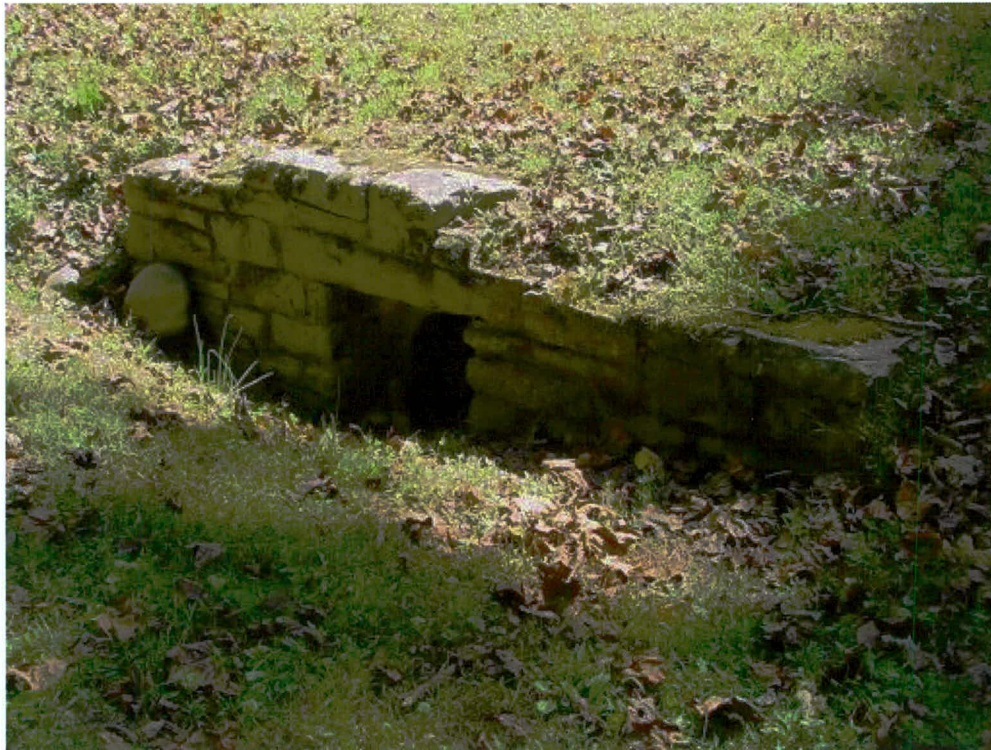
Figure 42. Pipe culvert (Sta 25+48) – north headwall, east of intersection with Big Cove Connector Road
