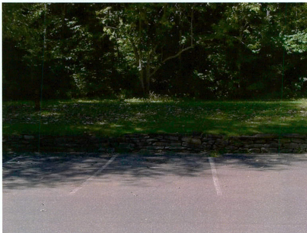
Figure 34. Detail, retaining wall in original visitor parking area at Oconaluftee Visitor Center, looking west to Newfound Gap Road
