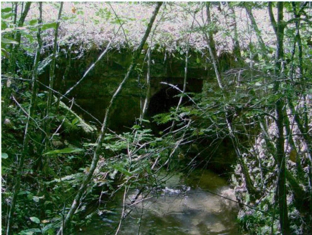
Figure 15. Pipe culvert (Sta 17+09) – east headwall, south of entrance to Smokemont Campground (west side not accessible for photography)
