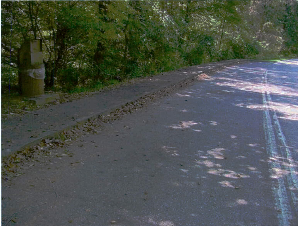
Figure 41. Automobile pull-out, south side Newfound Gap Road near intersection with Big Cove Connector Road
