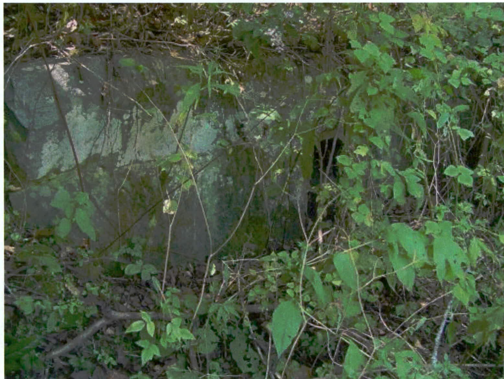
Figure 20. Pipe culvert (Sta 18+00) – west headwall, north of existing and proposed intersection with Tow String Road
