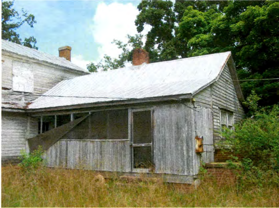
Plate 5. Cashion-Moore House, Rear (East) Elevation of Main Block and Rear Ell, Looking North.
