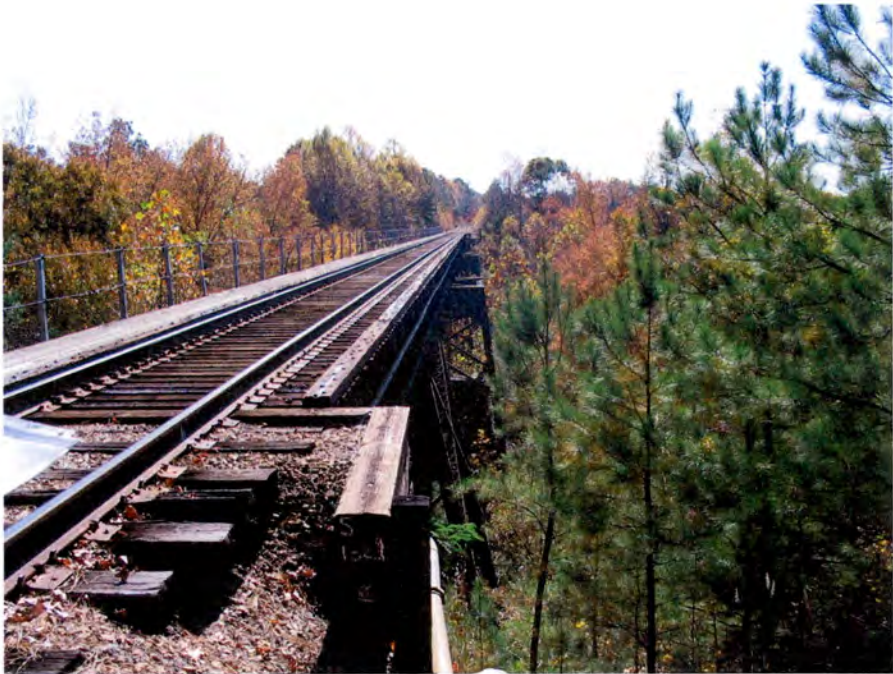
Plate 19. Seaboard Air Line Railway Bridge over Cedar Creek, Franklin County, Looking South.
