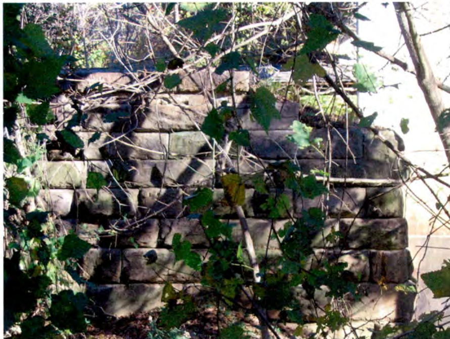
Plate 18. Raleigh and Gaston Railroad Bridge Piers at Crabtree Creek, Raleigh, Wake County.
