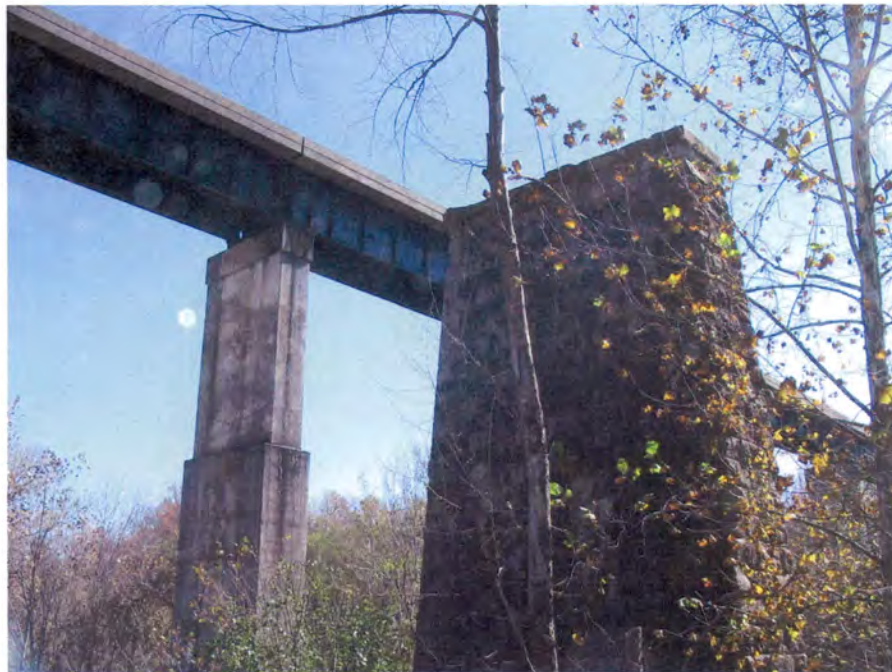
Plate 10. Raleigh and Gaston Railroad Bridge Piers at Tar River, Modern Seaboard Air Line Bridge in Background, Franklin County, Looking South.
