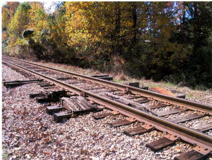
Plate 22. Seaboard Air Line Railway Defect and Dragging Detection Equipment at Cedar Creek, Franklin County.
