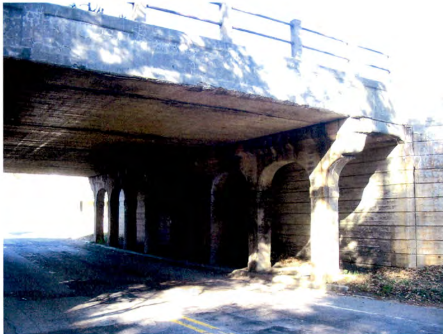
Plate 25. Seaboard Air Line Railway Bridge over U.S. 158, Substructure and Abutments, Norlina, Warren County.
