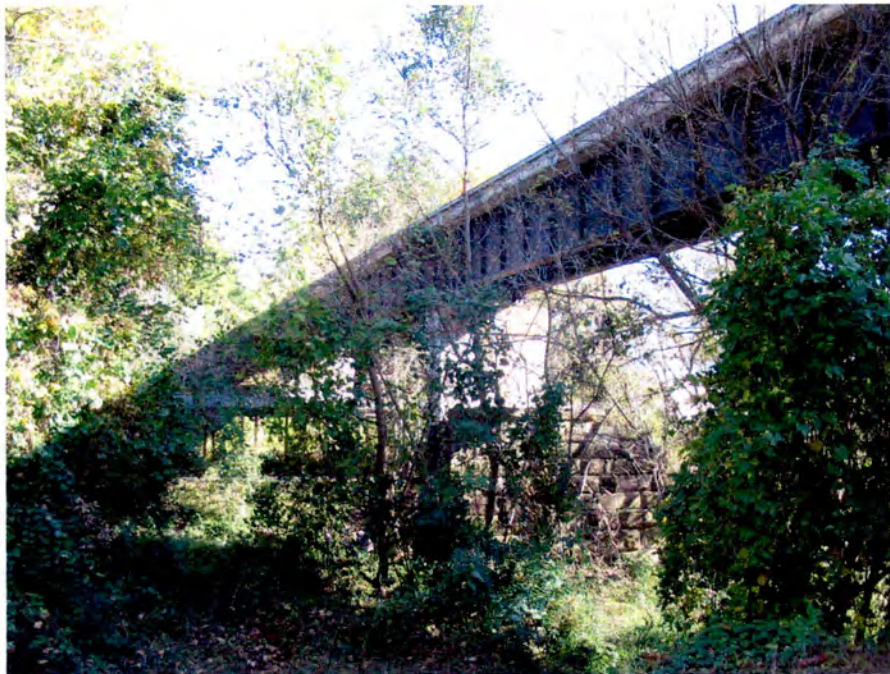
Plate 16. Raleigh and Gaston Bridge Piers at Crabtree Creek, Modern Seaboard Air Line Bridge Above, Raleigh, Wake County, Looking North.
