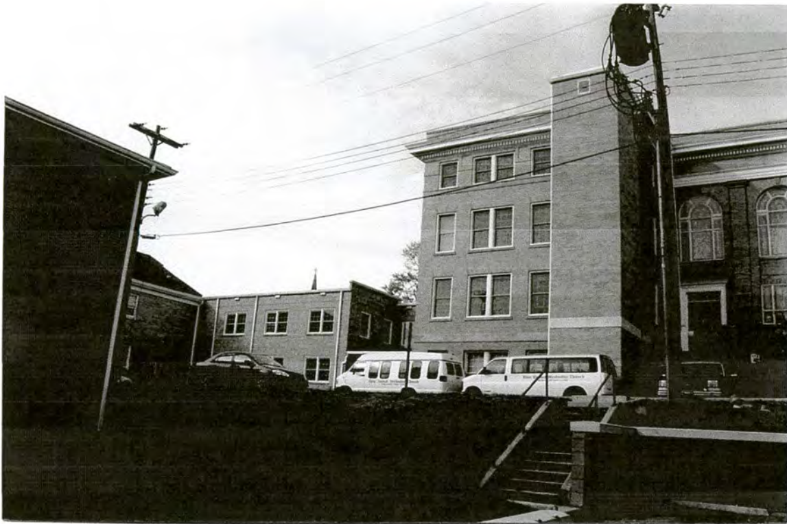
Plate 29: First United Methodist Church – original 1925 block, south side elevation, at right; 1990s/2000s addition at left
