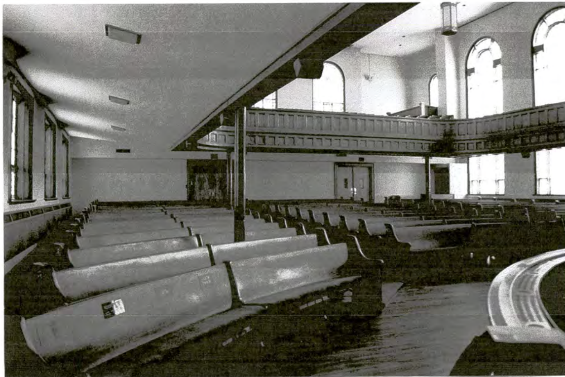
Plate 32: First United Methodist Church – sanctuary of original 1925 block, looking east from altar
