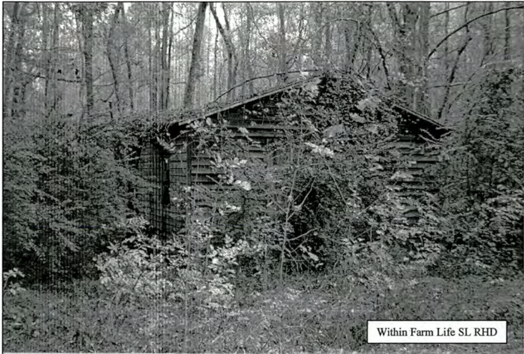
Property 6: Former Roberson Saw and Corn Meal Mill (MT 117, engine-powered) E. side NC 171, about 50 feet N of bridge Figure 23
