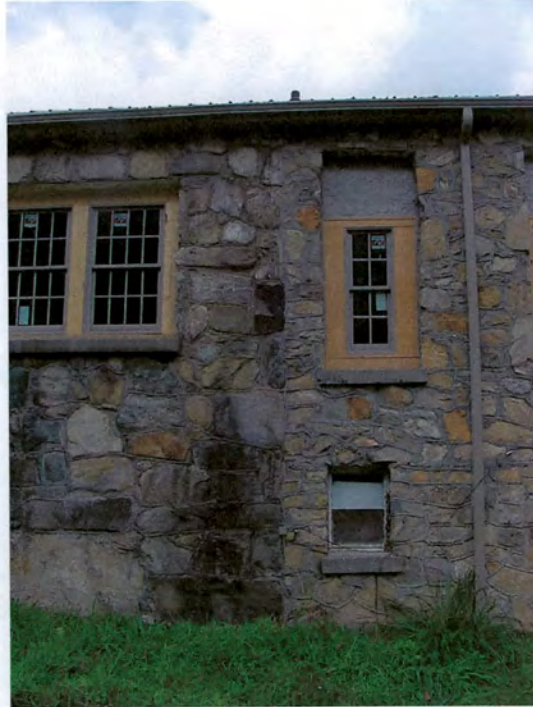
Ebbs Chapel School, detail, W end elevation of original building and 1950s wing (September 2004)
