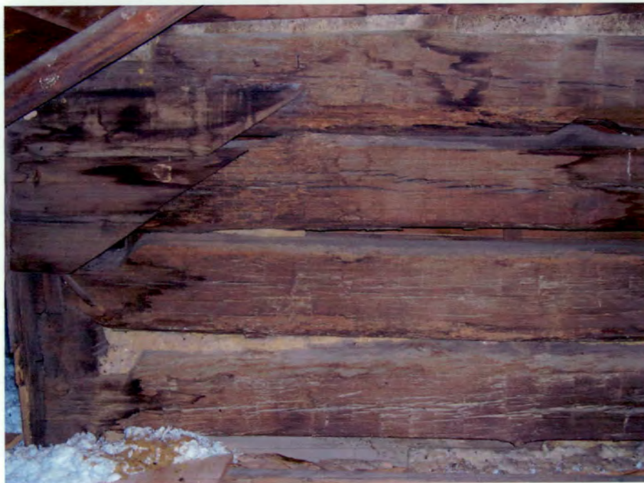
Exposed Log Wall (West Elevation of Original House) View from Kitchen Attic
