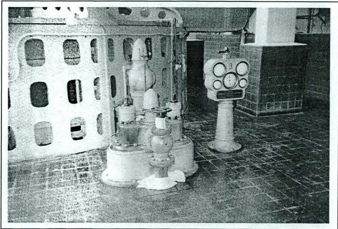
Figure 4.30. Rhodhiss Development, Rhodhiss Powerhouse; view of historic governor at generating unit #3; looking south-southwest.
