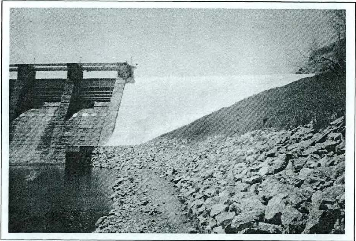
Figure 4.44. Oxford Development; view of new spillway at north end of dam; looking southwest.
