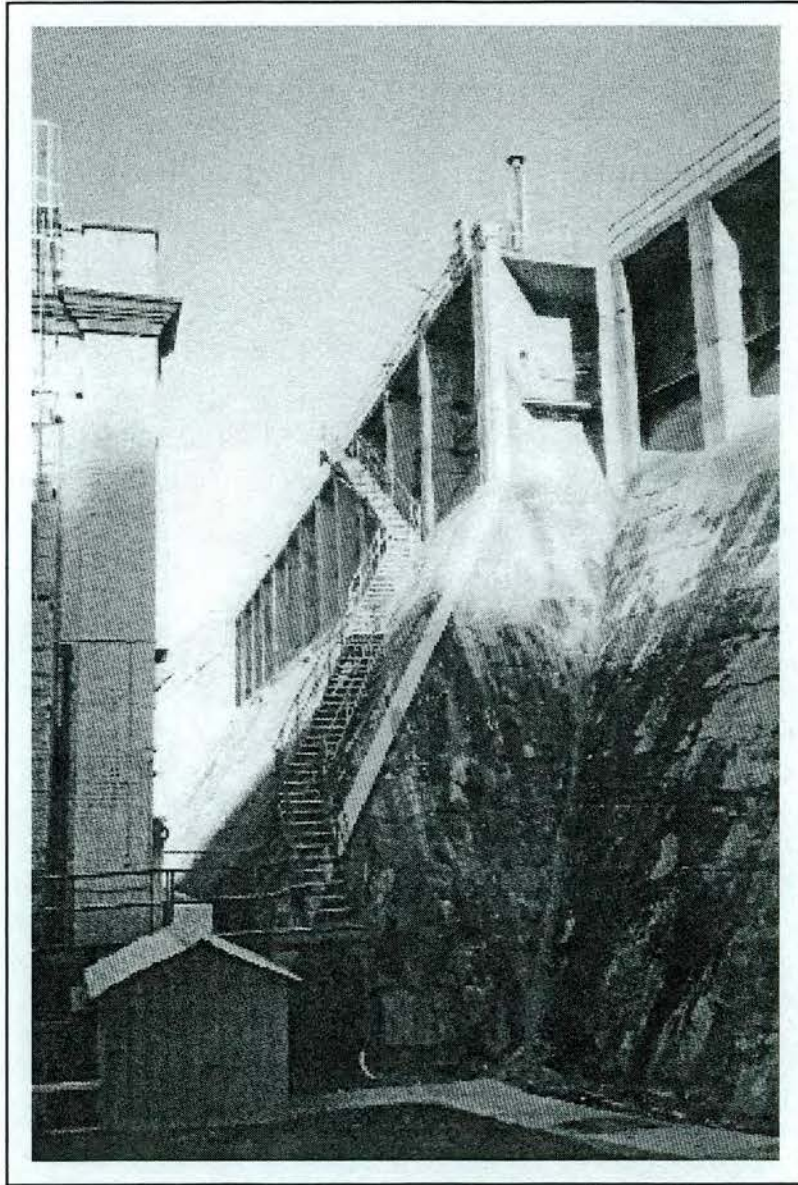
Figure 4.51. Lookout Shoals Development; view of dam/intake area to rear of powerhouse; looking west-northwest.
