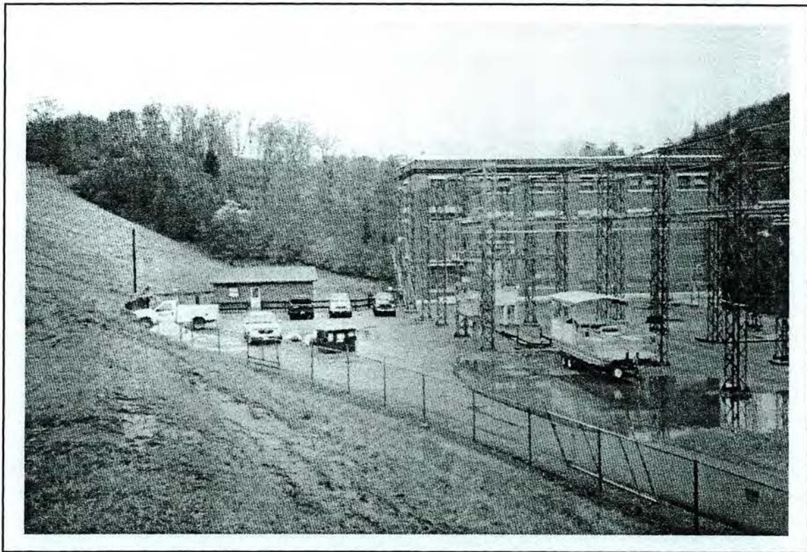
Figure 4.11. Bridgewater Development, Linville Powerhouse; view of office building, powerhouse (behind substation), and substation; looking northeast.
