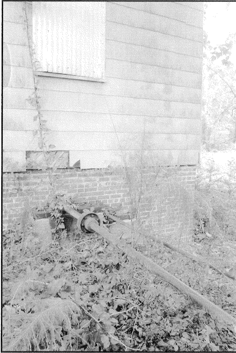
Figure 11. Shaft linking Turbine House (out of frame at right) to Grist Mill (shown in background). View to northeast.
