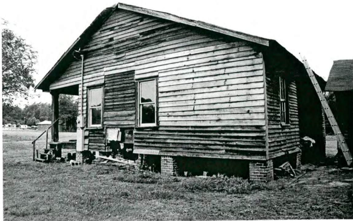
Plate 24: Calvin C. Gore House - south side and east rear elevations of house
