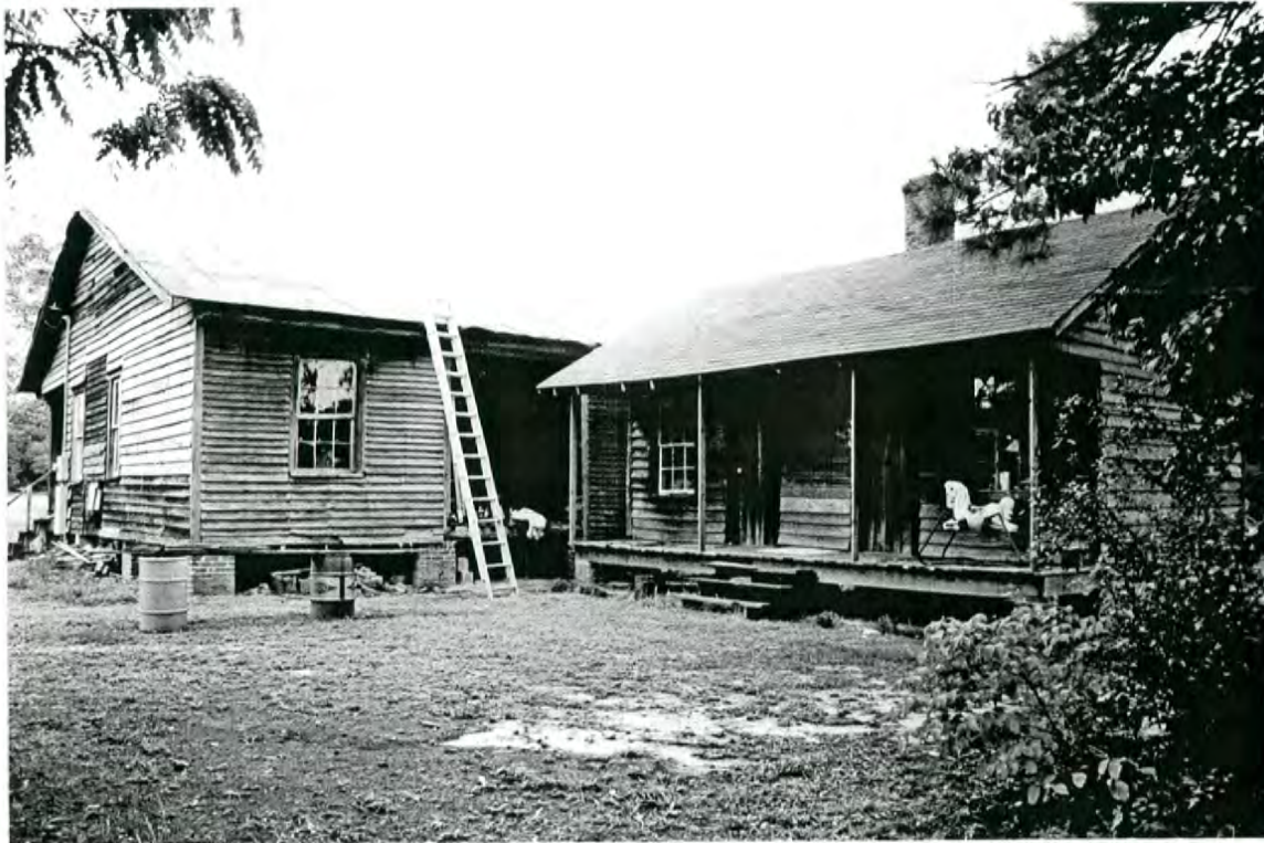
Plate 22: Calvin C. Gore House - east rear and south side elevations of house at left, kitchen wing at right
