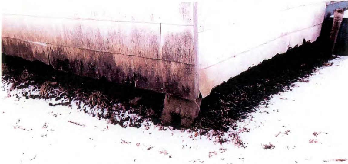
Plate 7. Laurel Hill Baptist Church – wood foundation piers
