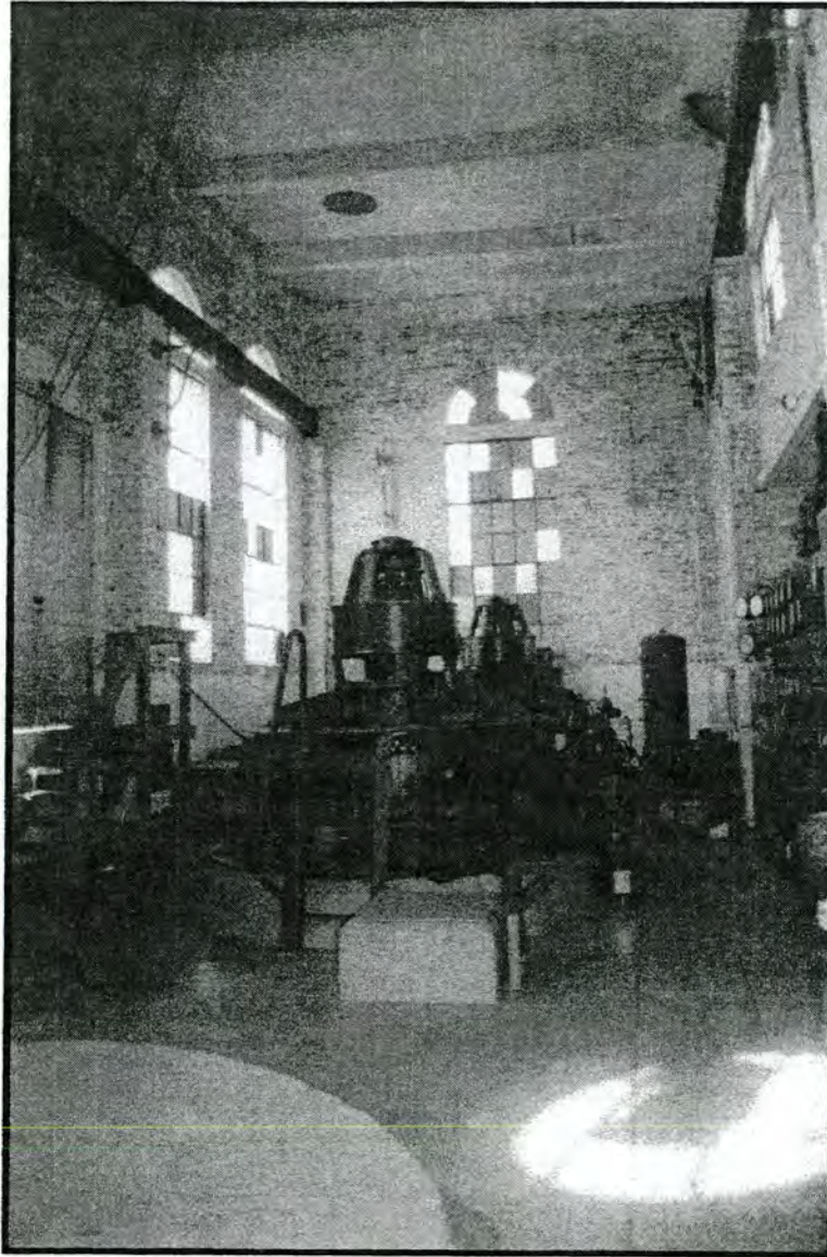
Figure No. 33. Interior view of the Franklin Powerhouse and original turbines.
