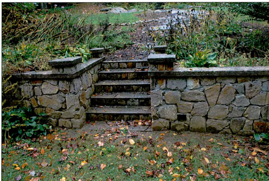
Figure 10: Garland House, steps leading to walkway, looking south. Katherine Husband, NCDOT, October 2011.
