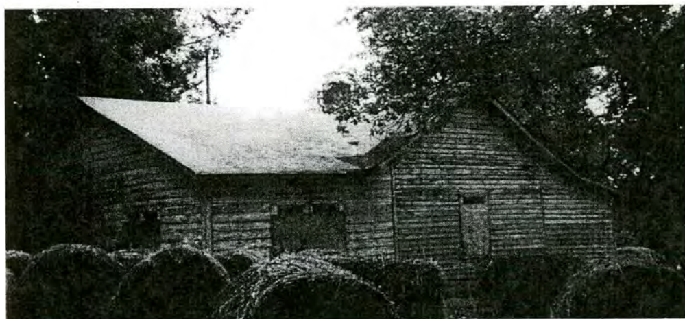
Figure 16: Property # 5 – C. L. Helms Tenant House North (back) and west (side) elevations. Photographed September 11, 2001.
