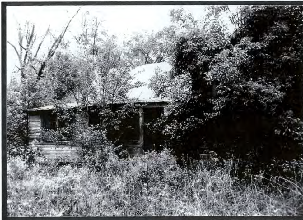
Plate V.29a Ervin Thomas House (#49) (UN385), Enclosed Shed- Roofed Addition Spanning West Elevation of Rear Ell
