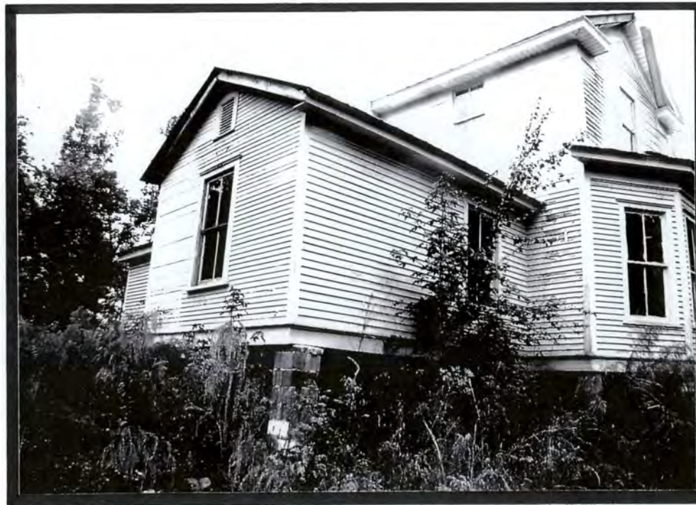
Plate V.25a Evans-Whitt House (#46) (UN113), Oblique, Ell on Rear (East) and Bay on North Elevations
