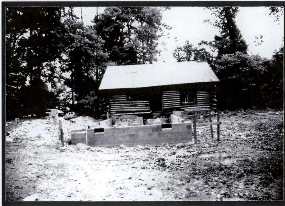
Plate V.10a Marcus Bruce Liles, Sr. House and Outbuilding (#2), Rear (Southeast Elevation), Foundation for Addition
