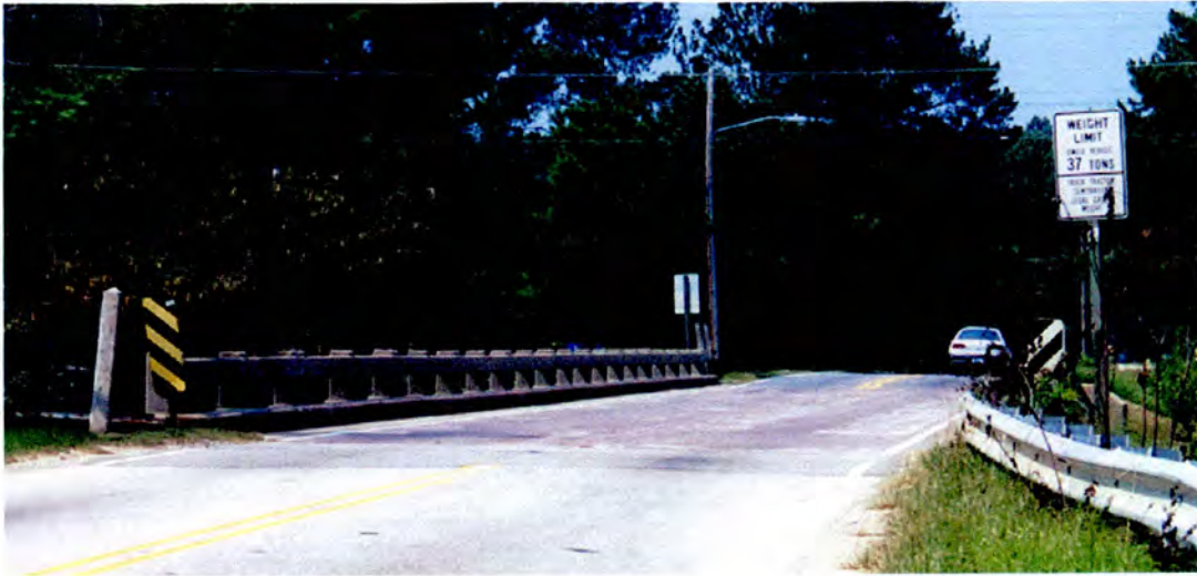
Figure 29. Property 8 - Bridge # 181. The property has been determined not eligible for the National Register because it is neither historically nor architecturally significant. Photographed September 11, 2002.
