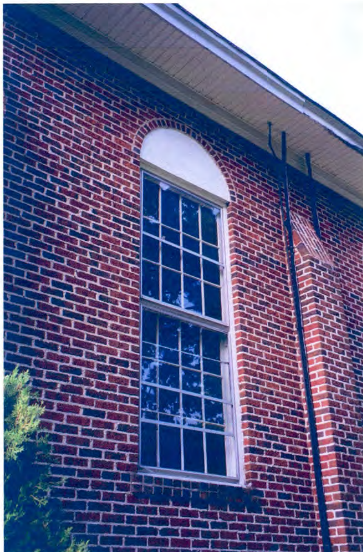
Figure 9. Falls of the Tar River Particular Baptist Church. Detail of window in north elevation. Photographed August 7, 2003.
