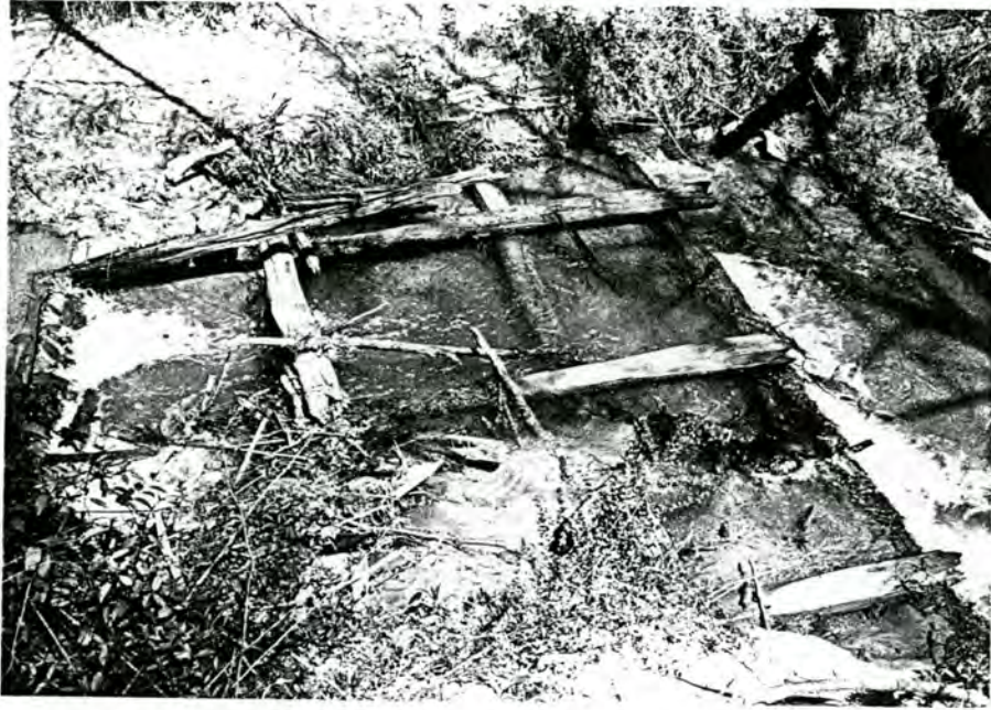
Plate 5. Remains of Stone Foundation and Framing Members of Mill Building in Canoe Creek Just Above J.D. Pitts Dam, Facing North Northwest from South Bank of Canoe Creek
