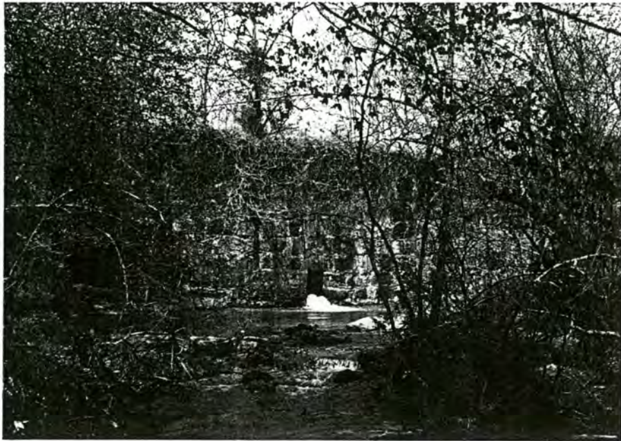
Plate 1. J.D. Pitts Dam, Facing West from the South Bank of Canoe Creek
