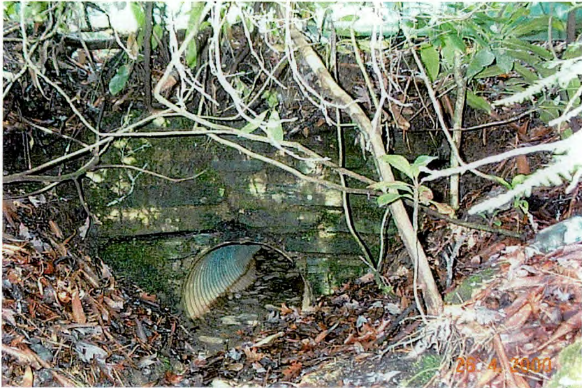
Plate 30: Small version, straight walled style. Note silt accumulation in culvert.
