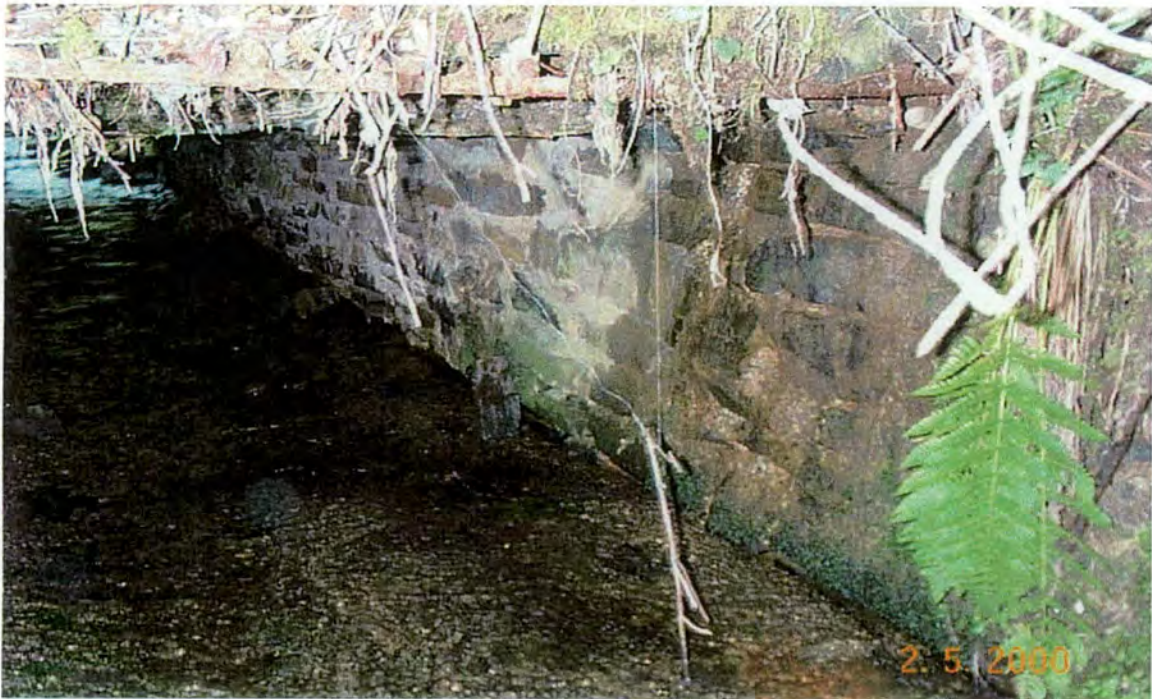
Plate 16: Close-up of upstream end of box culvert showing south side wall and exposed re-bar in concrete slab.
