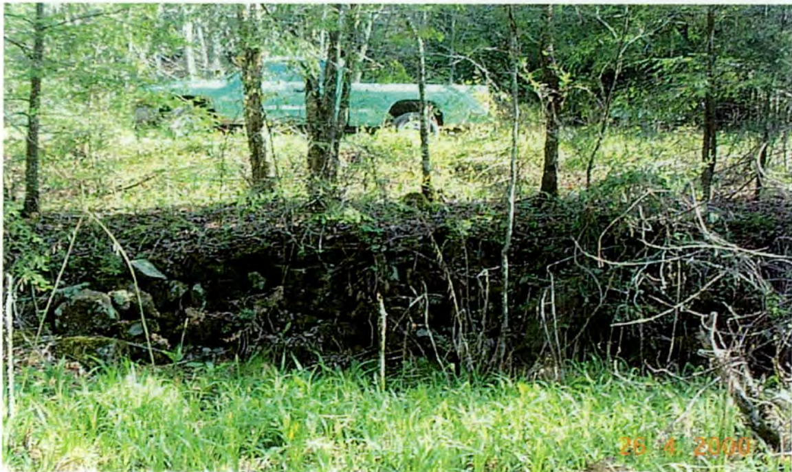
Plate 8: Northern section of retaining wall, view east. Buck Creek Road #350 is visible above.
