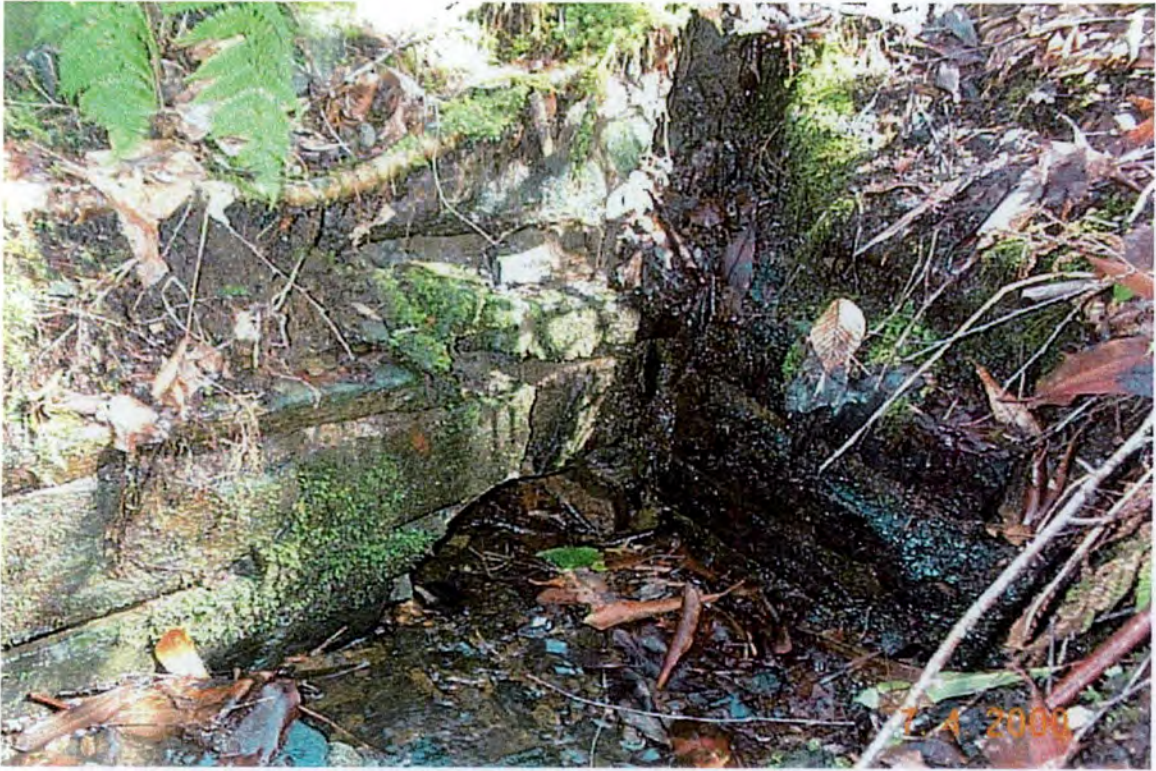
Plate 37: Winged corner style. Note silt accumulation in metal culvert.
