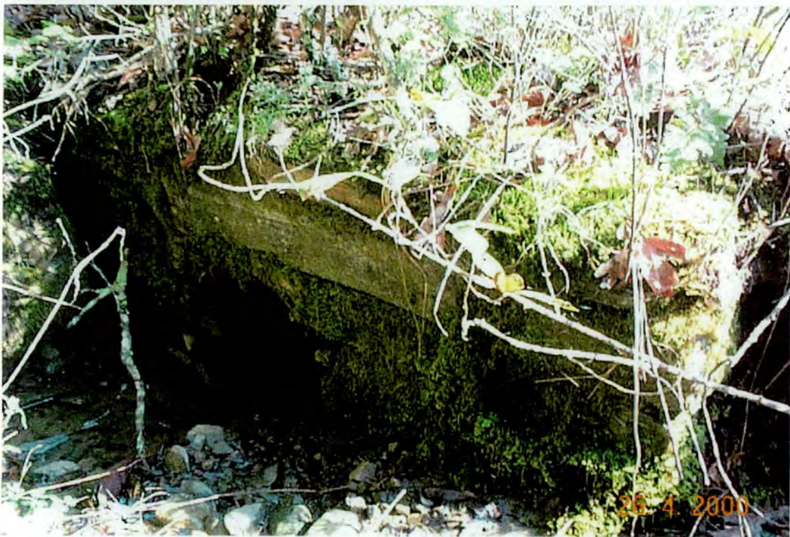
Plate 31: Small version, straight walled style. Headwall collapsing due to road grading.
