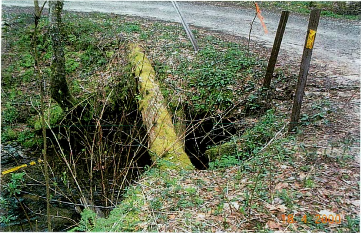
Plate 18: Downstream end of bridge showing erosion, view east.
