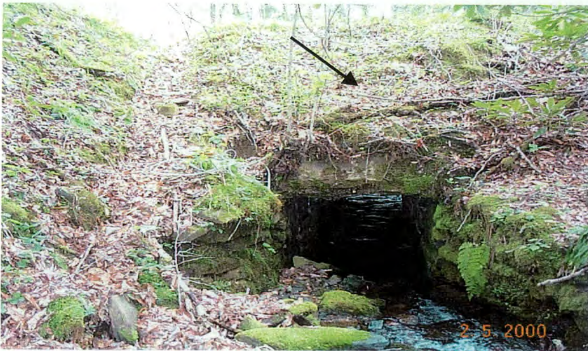
Plate 14: Downstream end of box culvert showing wingwalls. Arrow indicates fill over top of concrete slab (8 feet of fill).
