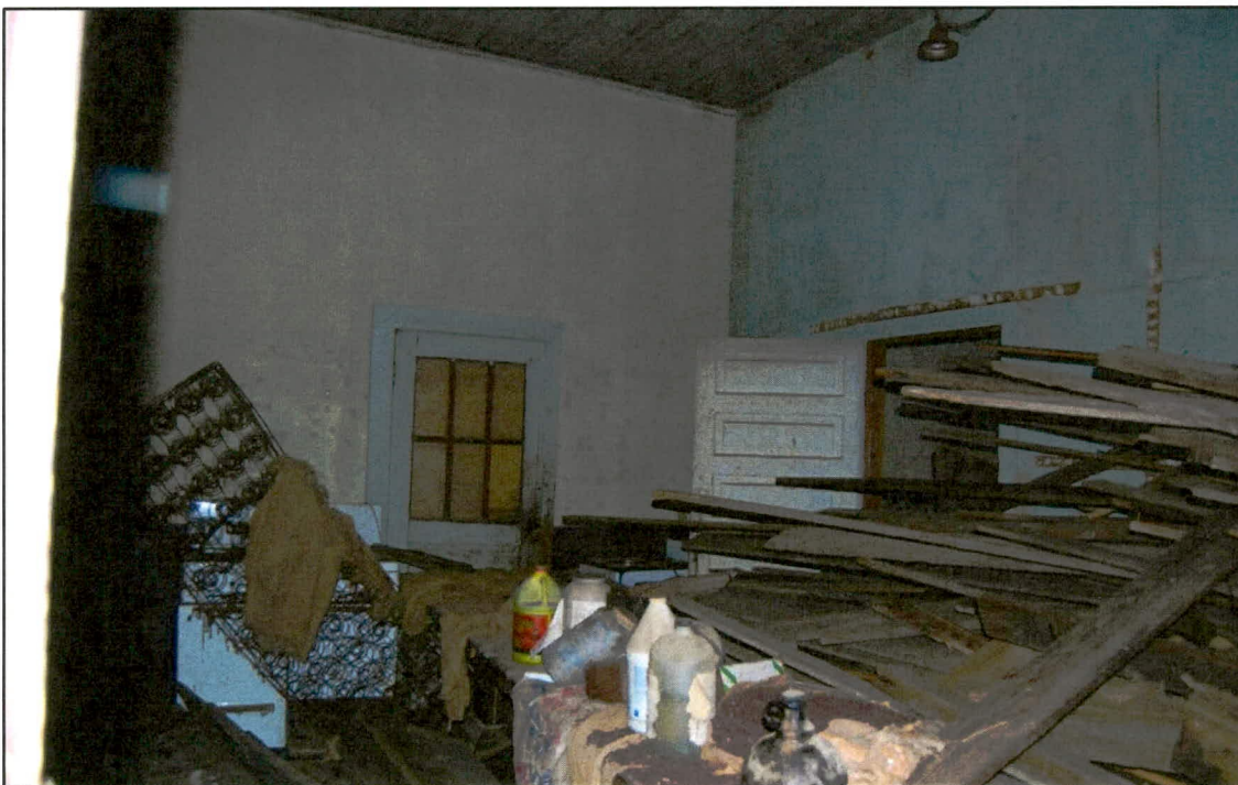
Figure 10. Ivey School: looking from entry in southern classroom toward gable-end wall with later entry at left and later partition wall with six-panel door at right; note original ceiling board in place at top and bit of brown wainscoting at far left beneath bed frame
