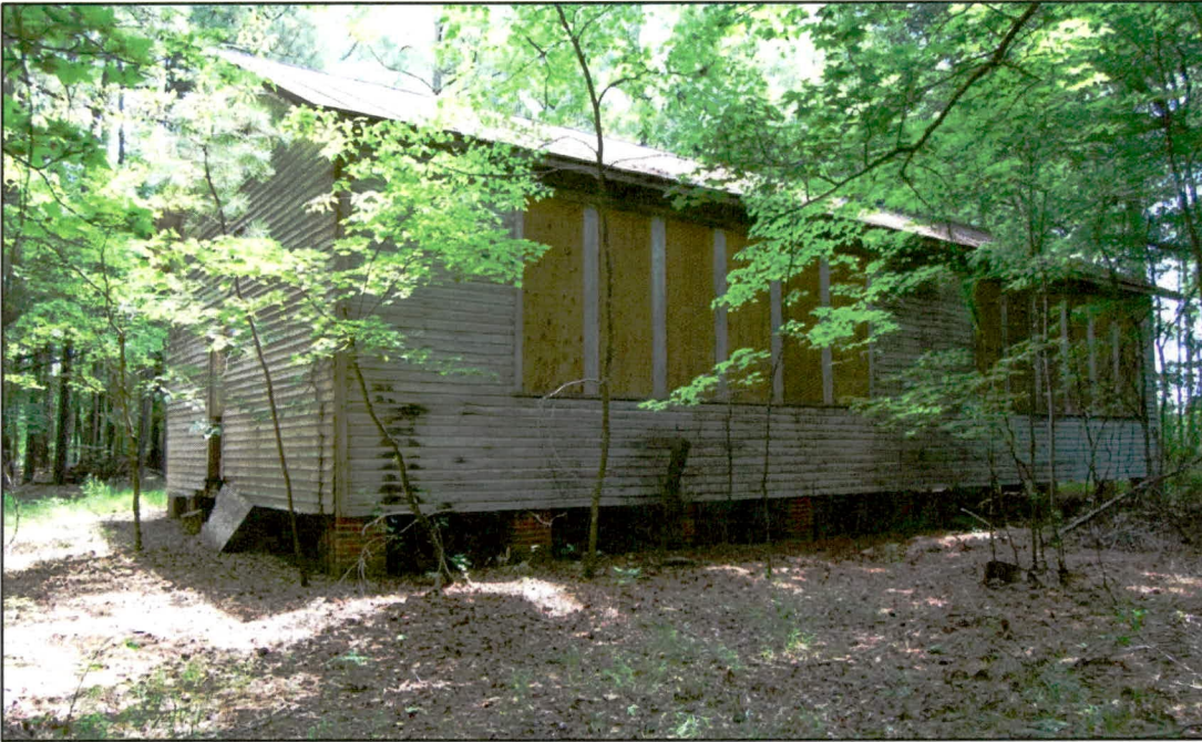
Figure 6. Ivey School: west rear and north side elevations; note original brick piers in place, boarded-over sets of classroom windows, and later added door at side elevation
