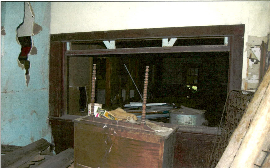
Figure 9. Ivey School: looking from southern into northern classroom from entry with original movable partition wall between classrooms at center and later-added, thin partition wall with holes punched in it at left; note intact wainscoting at original partition wall and at far northern gable-end wall
