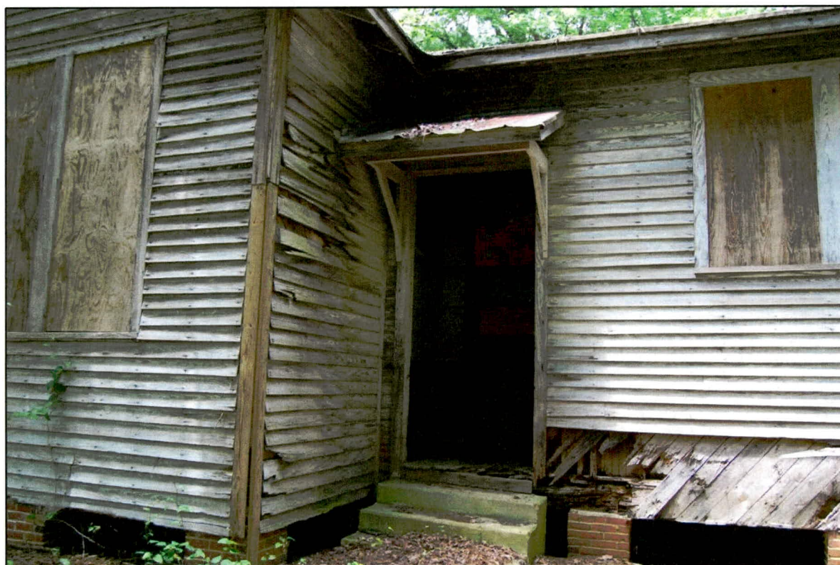
Figure 5. Ivey School: looking southwest at front elevation; note weatherboards and exposed sheathing at right, partially replaced cornerboards at left center, and entry with original triangular knee-braces, vestibule, wainscoting, and door at center
