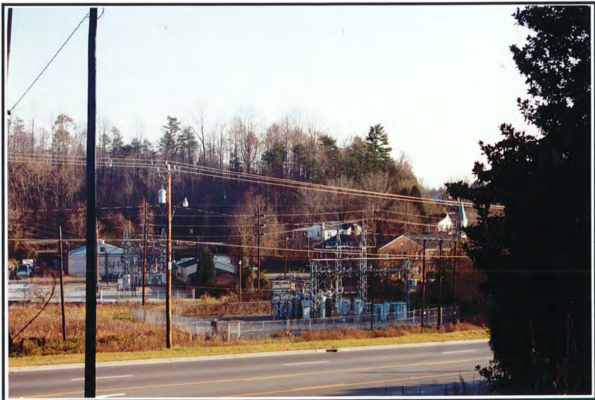
Photograph 56. View of transformer station visible from Structure 25, 26, 28, 31 and Streetscape 27, facing east-southeast.
