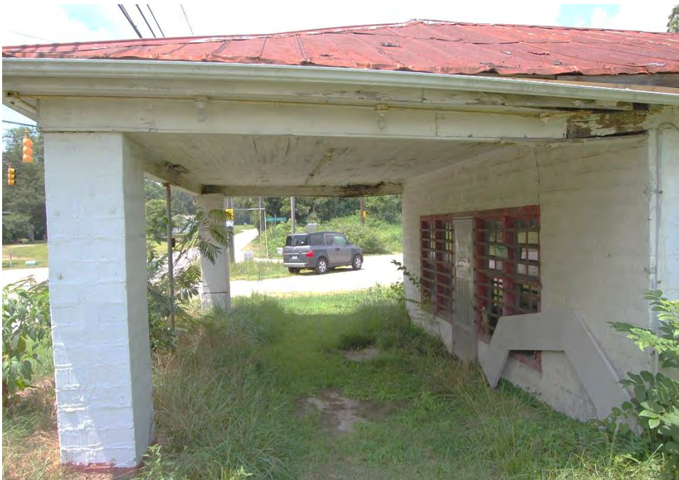
Plate 538. Auburn, Holland Smith Store (No. 272), Deteriorated Pump Canopy, Looking West.
