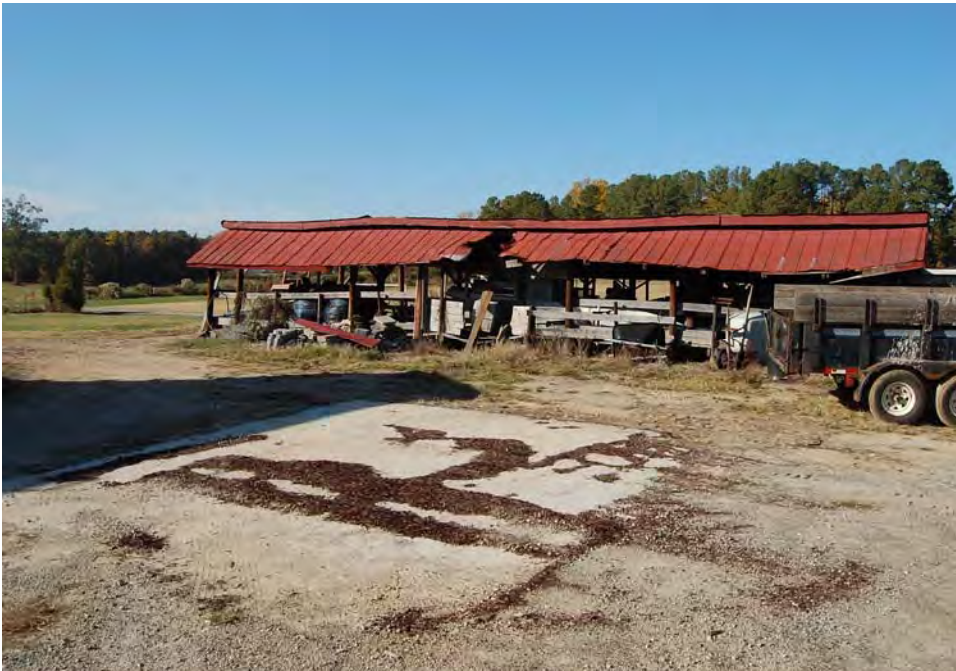
Plate 32. Pierce Farm, Equipment Storage Shed and Concrete Pad (Site of Destroyed Building), Looking North.
