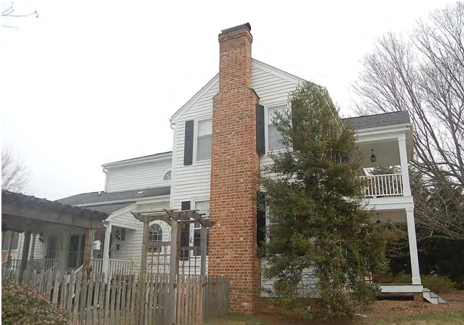
Plate 687. Burt-Utley House, Side (West Elevation), Rear Ell Additions, and Breezeway, Looking East.
