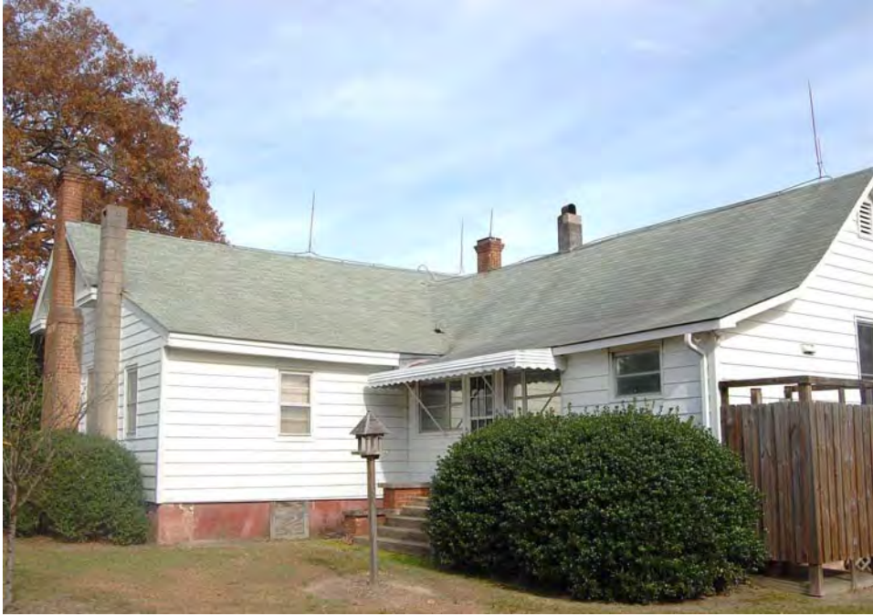
Plate 57. Bell-Pierce Farm, Eastern Tract, Bell-Pierce House, Rear (South) Elevation and Rear Ell, Looking North.
