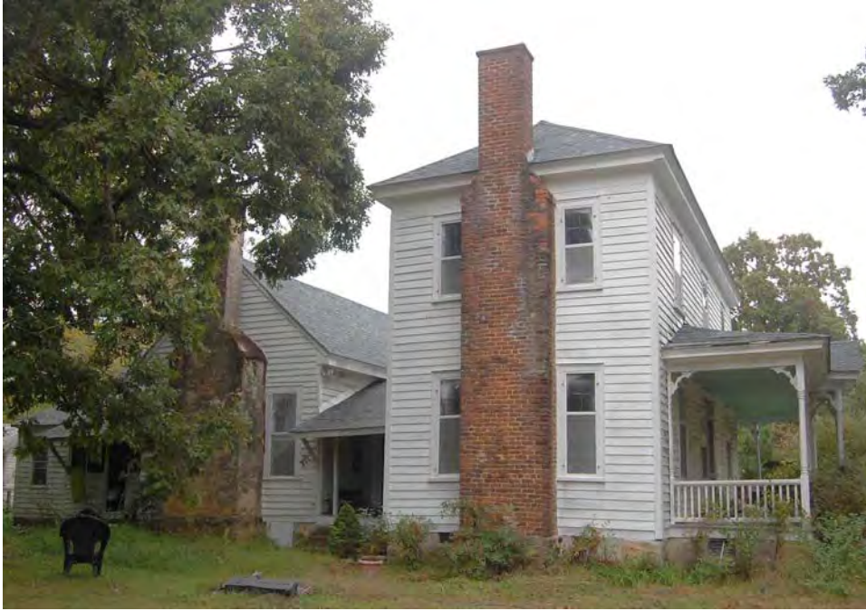
Plate 339. Baucom-Stallings House, Side (West) Elevation and Rear Wing (Original House), Looking East.
