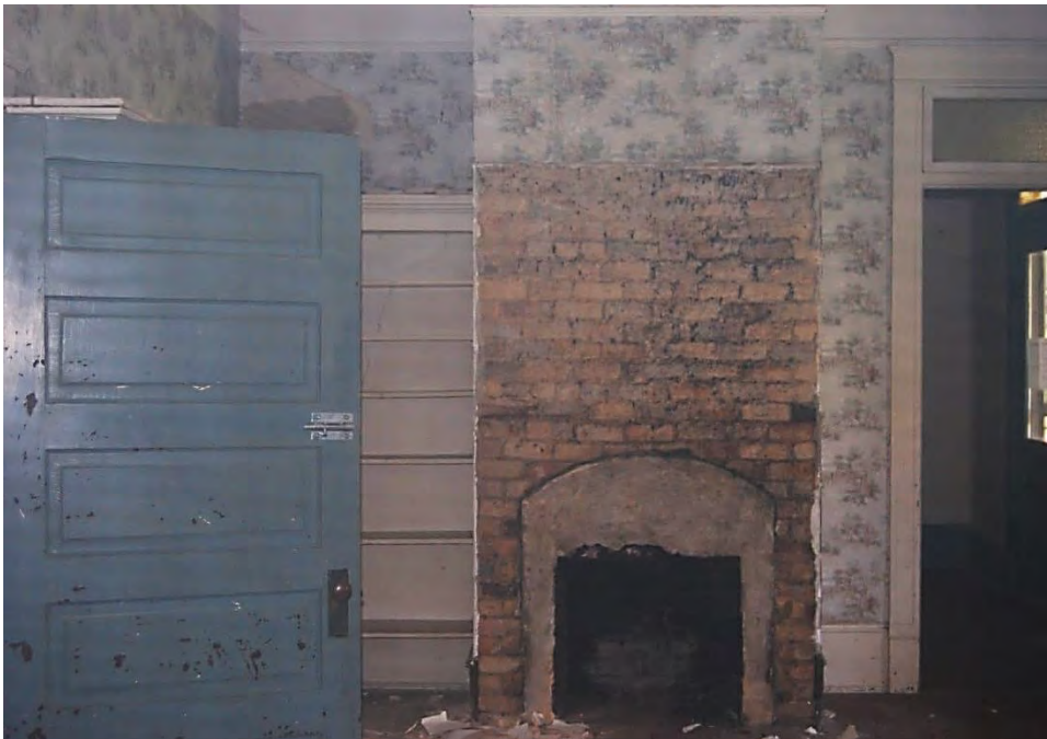
Plate 512. Johns-Lane-Poole House, Interior, Front East Room, Missing Mantel and Horizontal-Panel Door.
