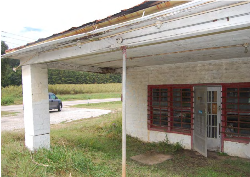
Plate 539. Auburn, Holland Smith Store (No. 272), Deteriorated Pump Canopy and Facade, Showing Makeshift Support and Deteriorated Pier, Looking Northwest.
