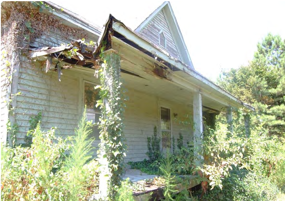
Plate 495. Tomlinson-Banks House, Façade and Ruinous Porch, Looking Southwest.
