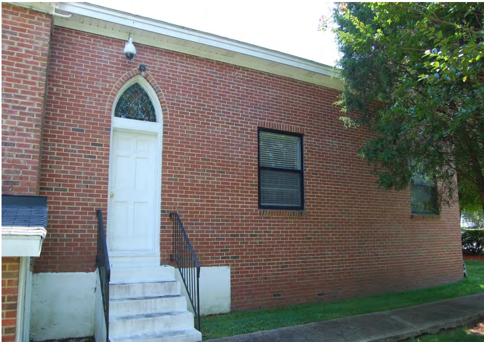
Plate 429. Popular Springs Christian Church, 1932 Church, Side (West) Elevation, at Junction with Modern Rear Addition.
