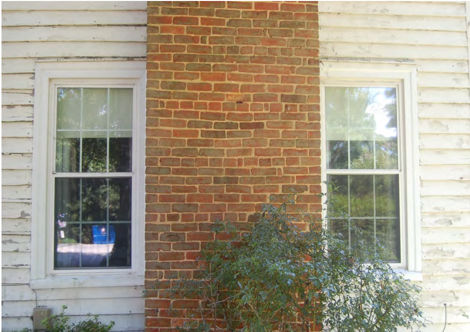
Plate 488. David Lewis House, Side (West) Elevation, Detail of Chimney, and Replacement Windows.
