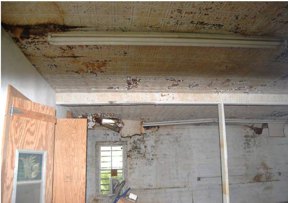
Plate 540. Auburn, Holland Smith Store (No. 272), Interior, Showing Deterioration and Rear Partition.
