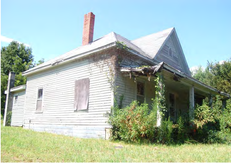
Plate 494. Tomlinson-Banks House, Façade and Side (East) Elevation, Looking Southwest From White Oak Road.
