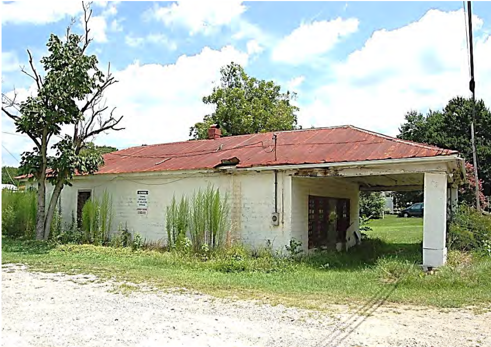
Plate 537. Auburn, Holland Smith Store (No. 272), Pump Canopy and Side (West) Elevation, Looking East.
