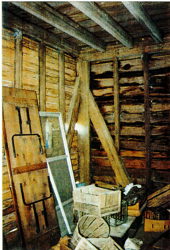
Figure 24: Warehouse (property 61), room 3, down brace
