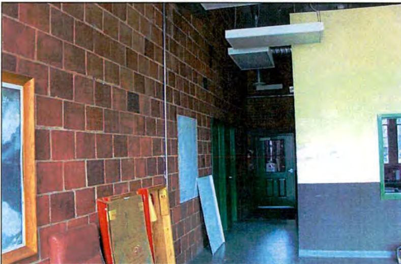
Interior clay tile wall, one of the only historic interior finishes noted during the site visit
