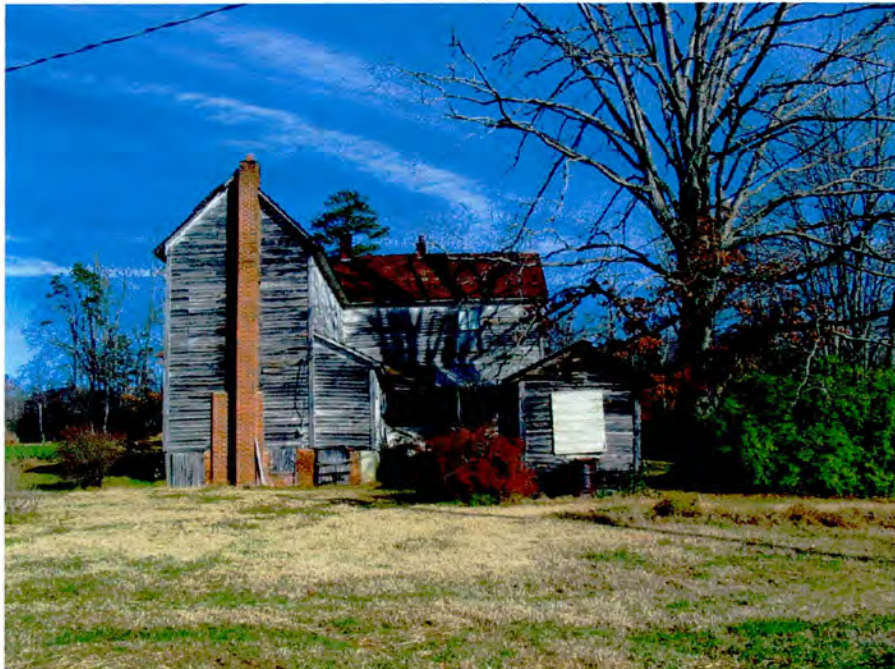
Plate 23. B.G. Hensley House, Rear (South) Elevation of House and Well House, Looking North.
