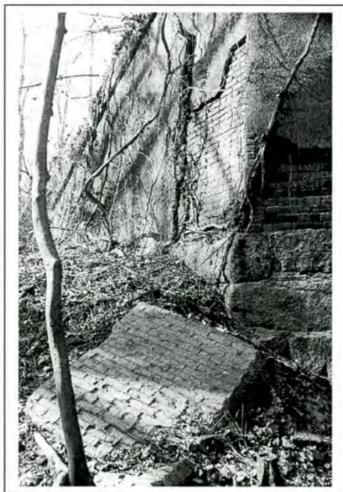
Figure 6. Detail of abutment on western riverbank. Detached section of concrete coating visible in foreground.
