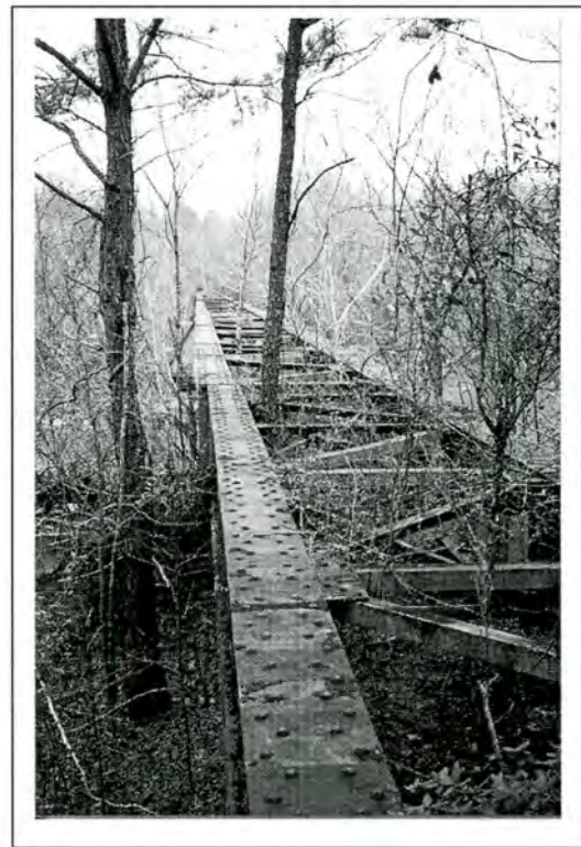
Figure 4. Deck looking west. Slight offset of swing span is visible in middle distance.
