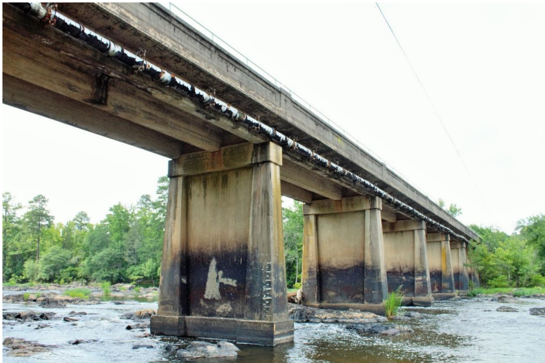
3. View from Haw River, looking northeast, showing ca. 1980 water pipe suspended from bridge
